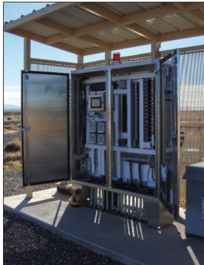
The wastewater system is controlled by an Orenco TCOM™ custom control panel. Photos courtesy of SCG Enterprises.
