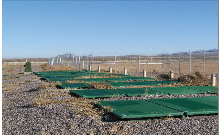
Eight AX100 pods treat widely-varying flows up to 30,000 gpd. Photos courtesy of SCG Enterprises.
