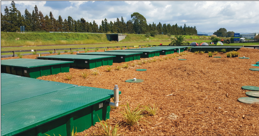
Installation and start-up of the AdvanTex treatment facility took place in only six weeks – in time for the start of the harvest and packing season that would bring an influx of seasonal workers.
